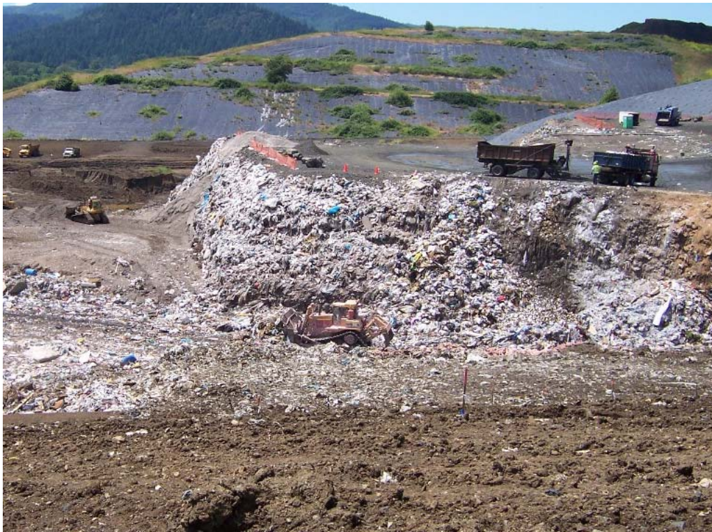
Figure 14. Landfill tip deck with near-vertical 10 m high tipping face with base liner in background.
