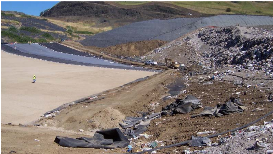
Figure 2. New MSW landfill cell on the left, tied into existing MSW cell on right and base liner system in background.
