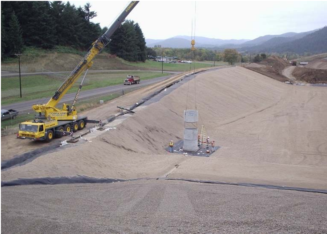
Figure 11. Setting below-grade vertical sump next to toe berm typical of landfill construction on base liner system.
