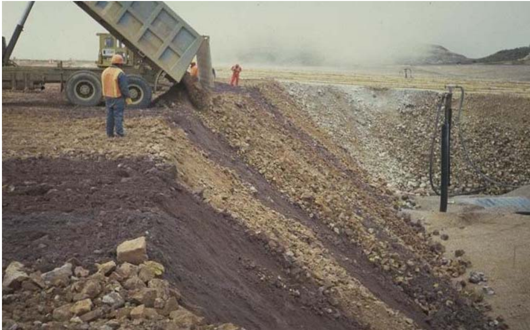
Figure 17. Angle-of-repose truck and dozer ore lift placement over lined leach pad. Rock boulders at toe of slope overlying base liner and protective drain fill cover layer.
