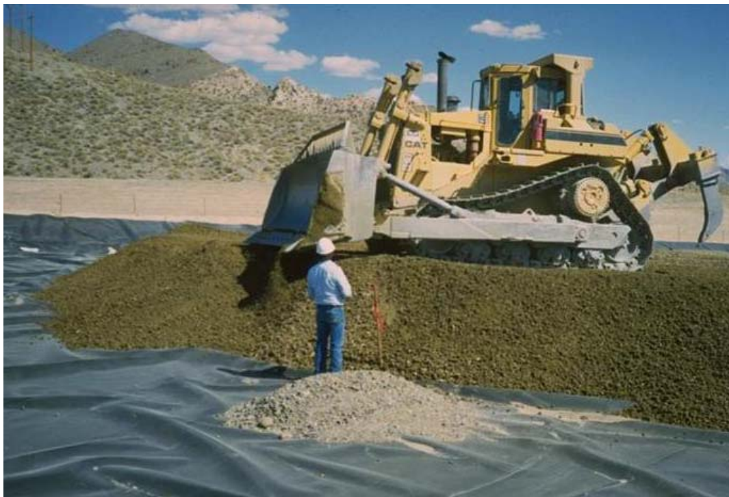
Figure 8. Typical drain layer placement over heap leach pad base liner. Landfill construction typically would be similar with thinner drain layer thickness and smaller dozer equipment size.
