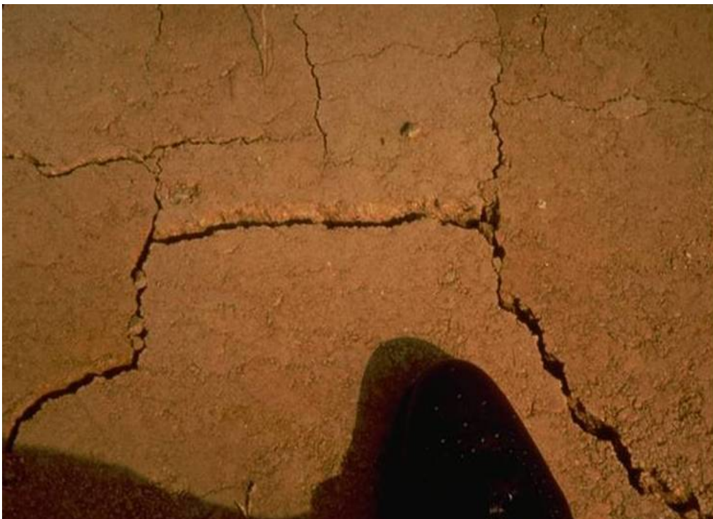
Figure 10. Desiccation cracks in exposed clayey soil liner 1 week after being placed wet of optimum moisture. Shoe toe shown in foreground for reference.
