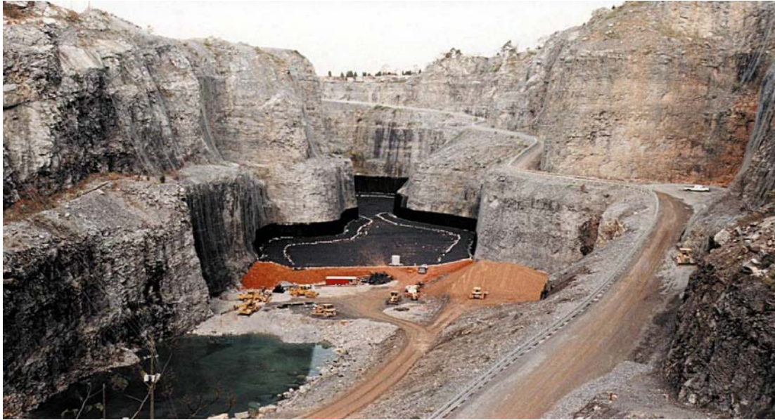
Figure 3 – Bristol landfill liner construction in open pit quarry with conventional composite compacted clay and geomembrane across the valley floor. Note groundwater conditions shown in the bottom right side below the landfill liner system.
