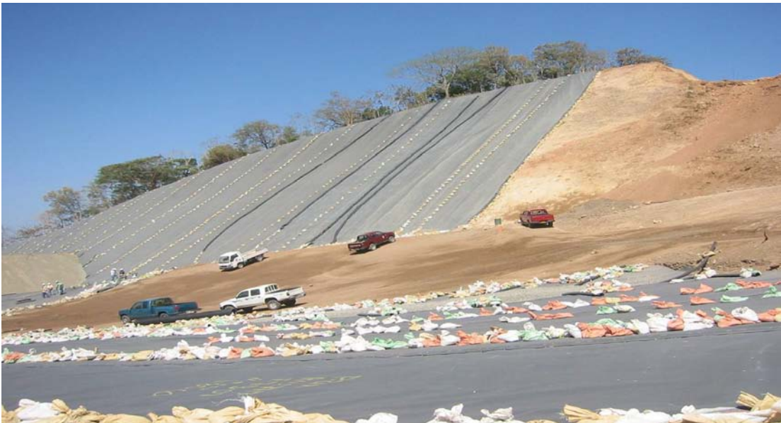
Figure 2 – Steep valley wall lined with composite geosynthetic clay liner (GCL) and geomembrane and valley floor being prepared with conventional compacted clayey soil liner in preparation for geomembrane liner installation.
