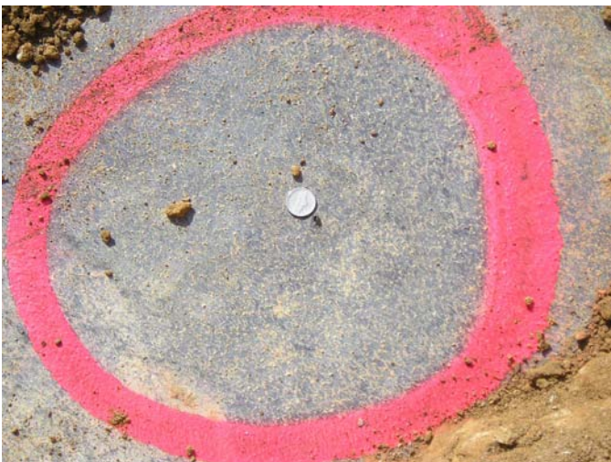
Figure 6. Small puncture found under approximately 1.0 m of soil at Site 1
