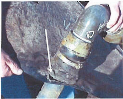
(a) Failed pipe boot at skirt-to-sleeve weld.
