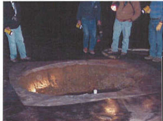
(b) Sinkhole at bottom of reservoir caused by failed pipe boot.
