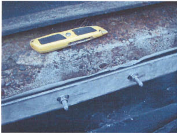
(a) Thick fuel-resistant moldable sealant used to provide leak-resistant seal against rough concrete.
