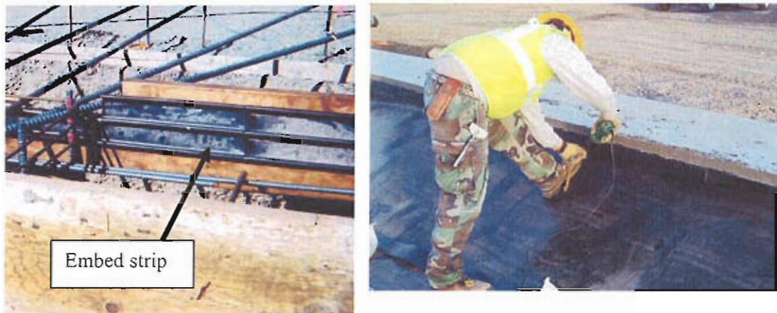
(a) Embedment strip nailed to inside of forms for secondary containment in haz-waste building.
