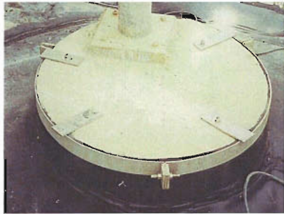
(d) Heavy wide custom clamp around end of a penetration.
