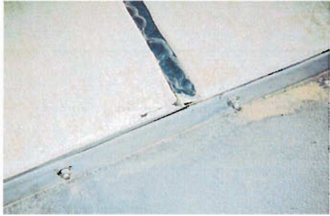
(b) Bad concrete joint will defeat batten when submerged.
