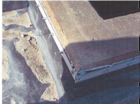
(d) Battens at corners need special attention. This one is missing a needed bolt.
