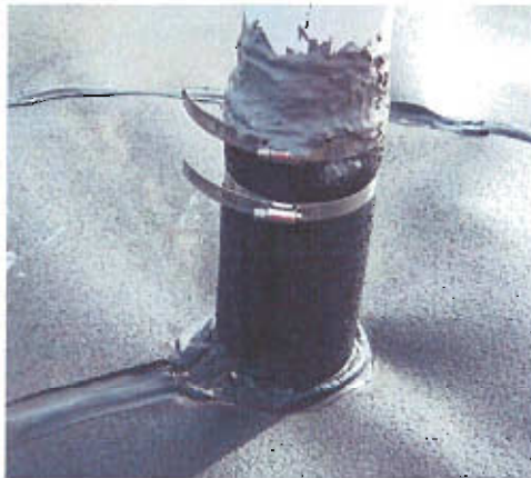
(a) Gasketed and banded boot with polysulfide coating on the end of the boot.
