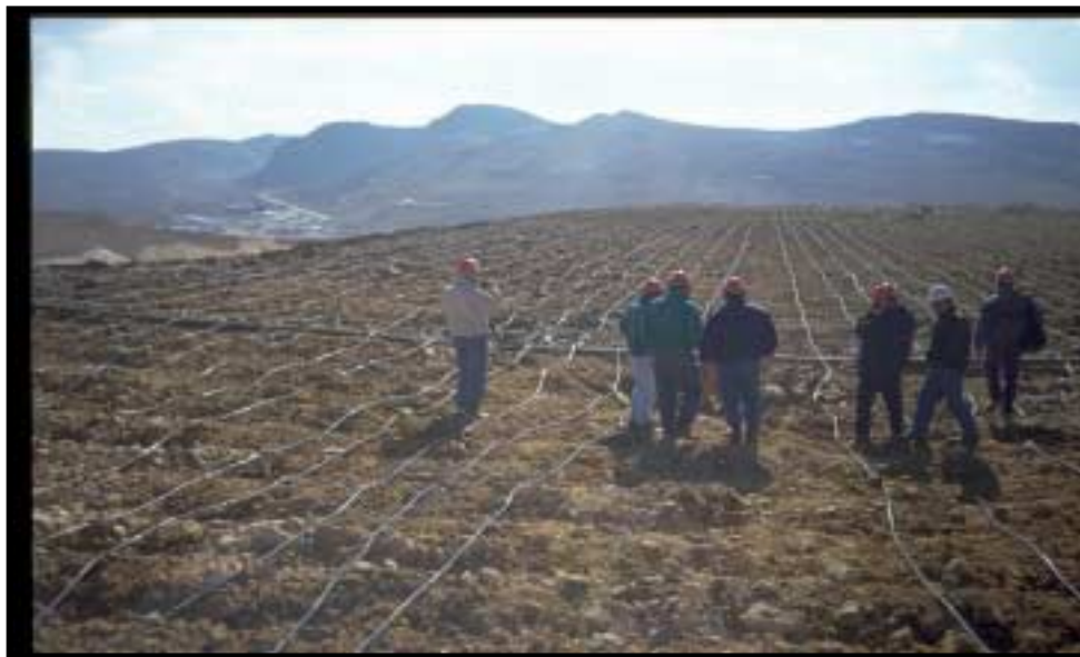
Photo 4 – Heap Leaching with Drip Emitters on Ore Surface (Northern Peru)
