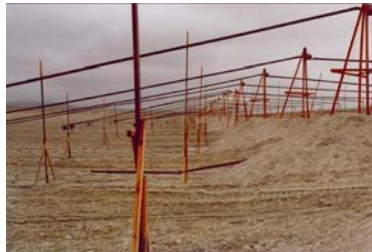
Fig. 2: Hydro-cyclone towers for underflow tailings beach development
