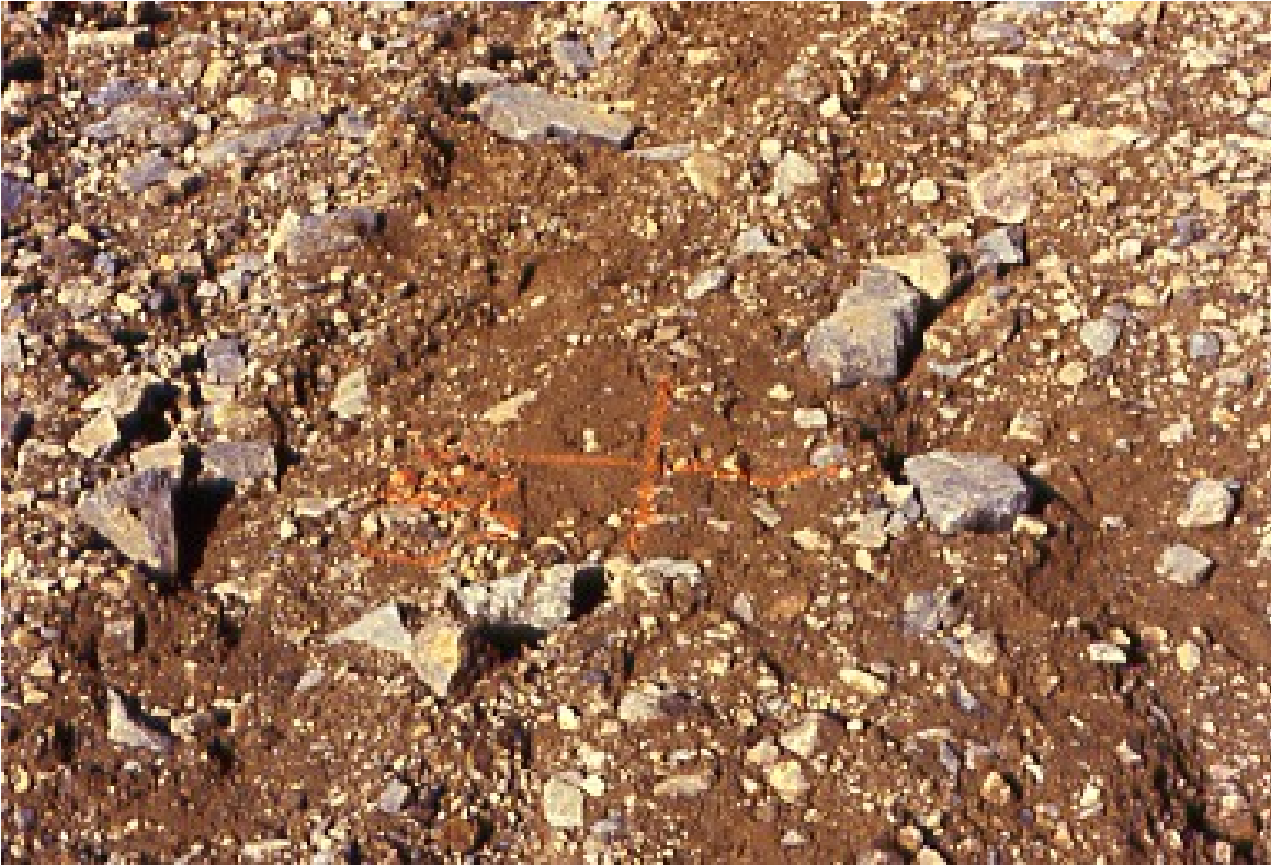
PHOTO 5 – INITIAL ROUGH TEST FILL SURFACE BY DOZER MARKED FOR SURVEYED MEASUREMENT AT 5 LOCATIONS ON ROCKFILL SURFACE
