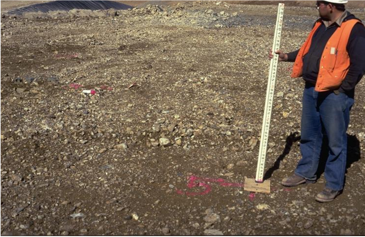
PHOTO 6 – TEST FILL CONTROL POINTS CROSS-MARKED FOR SURVEY AND SPACED 1 ROLLER WIDTH APART FOR CENTERLINE COMPACTION
