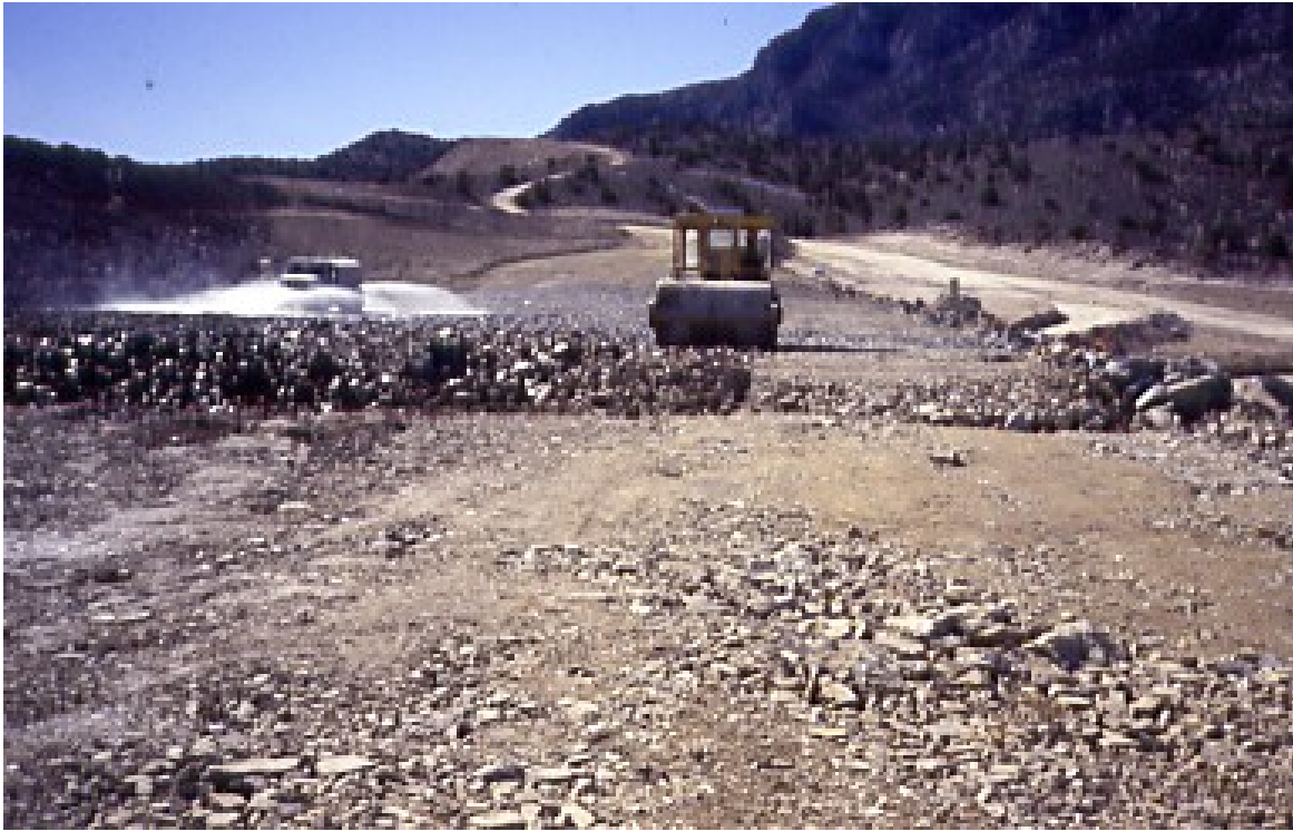
PHOTO 2 – WETTING AND COMPACTING 2 FT (0.6 M) THICK LOOSE ROCKFILL LIFT WITH 20 TON VIBRATORY COMPACTOR ROLLER
