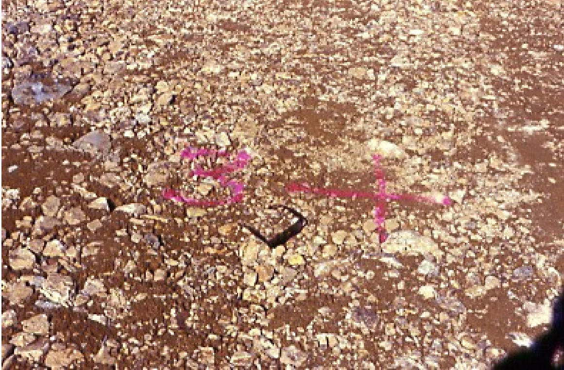
PHOTO 8 – TEST FILL SURFACE BECOMES MORE LEVEL WITH EACH PASS OF THE VIBRATORY COMPACTION ROLLER
