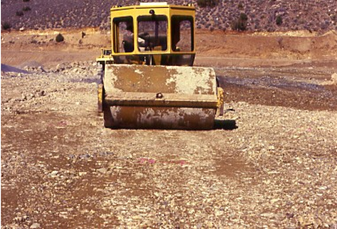
PHOTO 7 – TEST FILL SETTLEMENT POINTS ARE REMARKED FOR SURVEY AFTER 2 VIBRATORY COMPACTION ROLLER PASSES
