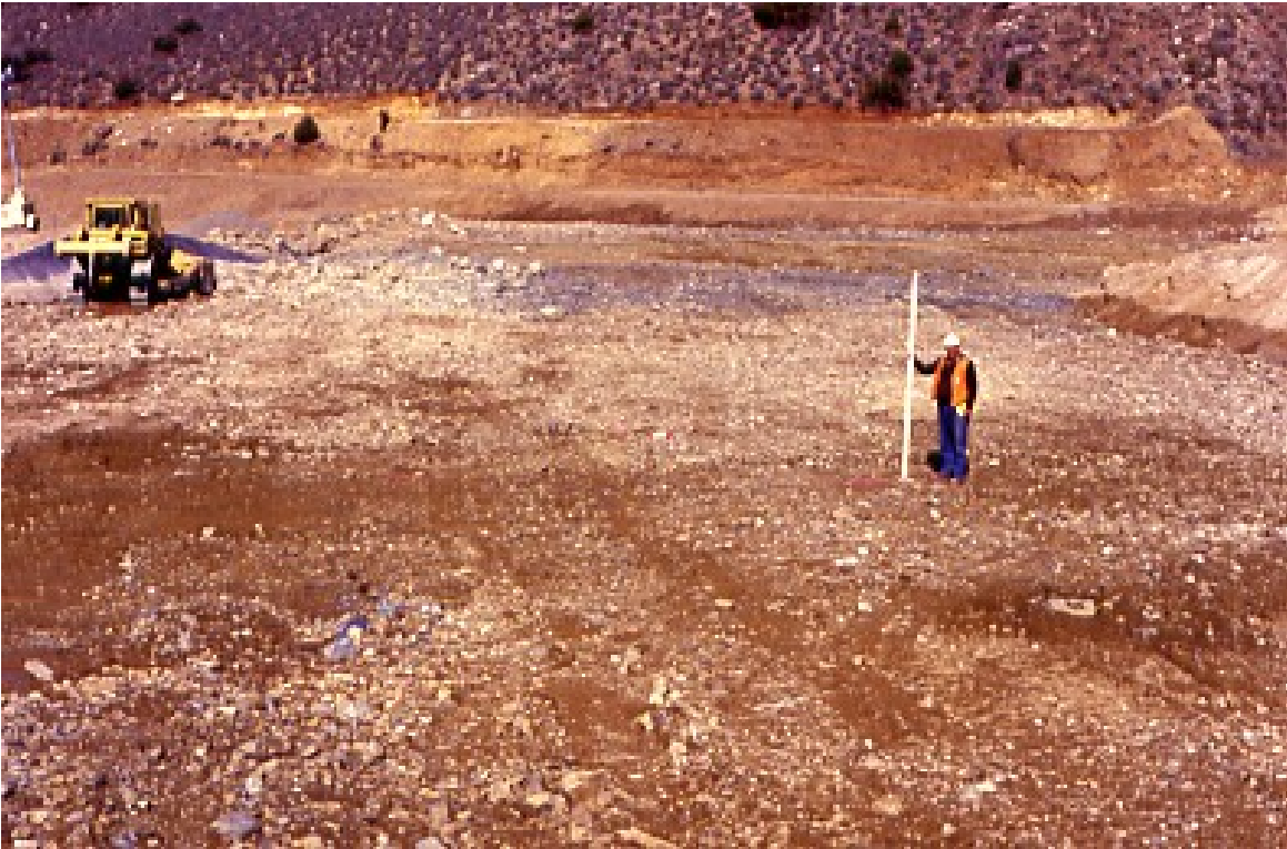
PHOTO 4 – INITIAL SURVEY MEASUREMENT OF LOOSE LIFT SURFACE ELEVATION IN TEST FILL (NOTE ROUGH ROCKFILL SURFACE)
