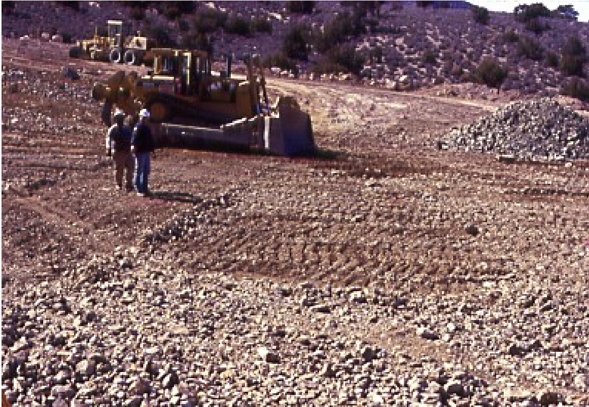
PHOTO 3 – DOZER PREPARED TEST FILL SURFACE FOR CONTROLLED ROLLER PASS VERSUS SETTLEMENT MEASUREMENTS IN 2 FT LIFT
