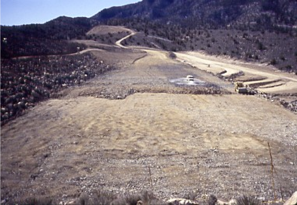
PHOTO 1 – ROCKFILL DAM CONSTRUCTION IN SOUTHERN CALIFORNIA WITH 50 FT (15 M) DOWNSTREAM RAISE TO EXISTING DAM
