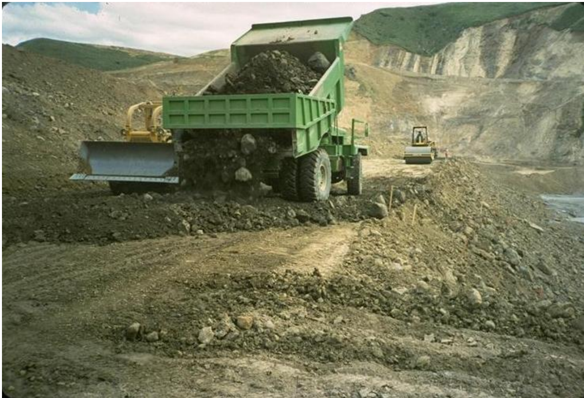
PHOTO 8 – HAUL TRUCK DUMPING MINUS 1 FT (0.3 M) TYPICAL ROCKFILL FRAGMENTS FOR DOZER PLACEMENT AND VIBRATORY ROLLER
