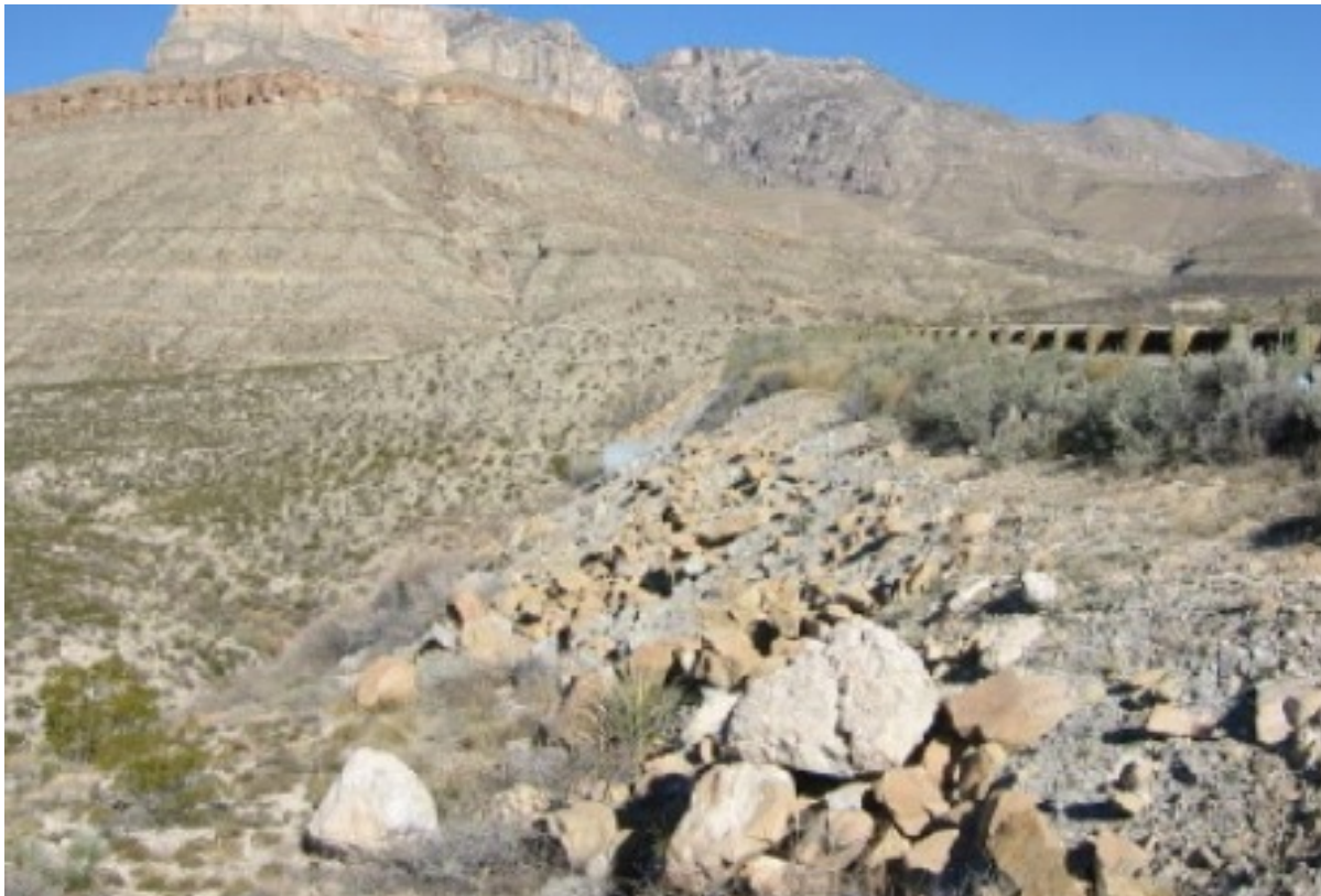
PHOTO 4 – HIGHWAY FILL SLOPE SHOWS AN UPWARD TRANSITION FROM ROCKFILL TO EARTHFILL MATERIALS FOR HIGHWAY SUBBASE
