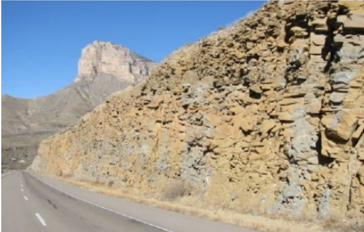
PHOTO 3 – ROCK BORROW DEVELOPMENT IN HIGHWAY CUT USED DRILL AND BLAST TECHNIQUES TO EXCAVATE AND REMOVE ROCKFILL MATERIALS
