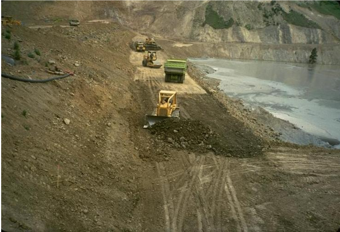
PHOTO 7 – ROCKFILL PLACEMENT ON UPSTREAM FACE OF 470 FT (143 M) HIGH EARTH AND ROCKFILL TAILINGS DAM
