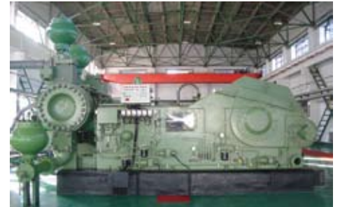
Top High-pressure choke/valve station
