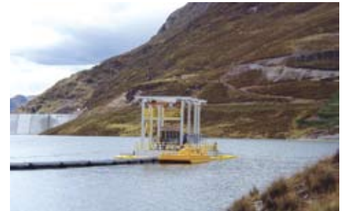
Top Copper tailings cyclone station
