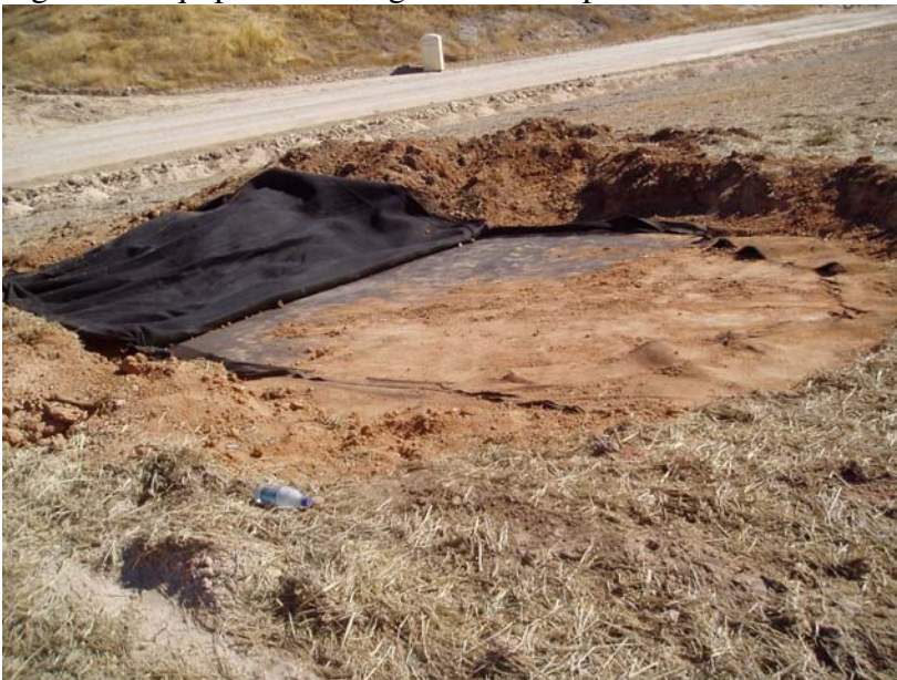
Figure 5. Equipment damage on side slope of Site 1
