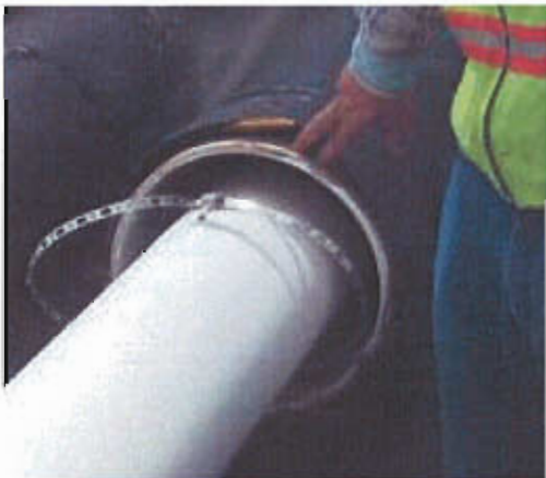
(c) Thin band clamp that has loosened and come off.
