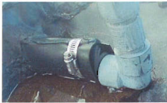
(a) Classic example of poorly constructed boot that violates all good construction principles.
