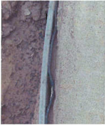
(a) Wavy substrate will cause leaks.
