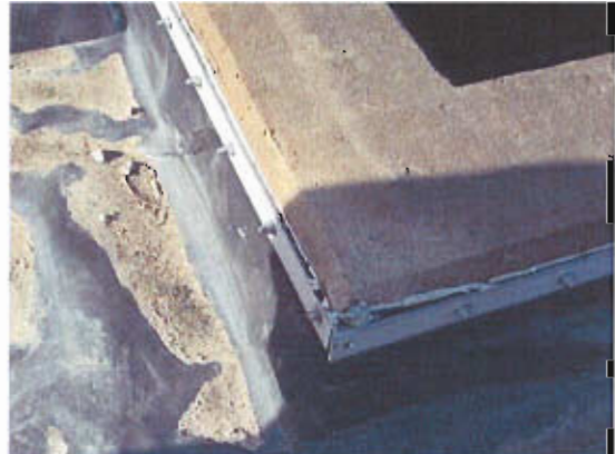
(d) Battens at corners need special attention. This one is missing a needed bolt.
