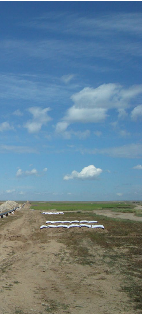
Bao Tou (Bai Yun E Bo) Iron Concentrate, Water and Thickened Tailings Systems, under construction, China
